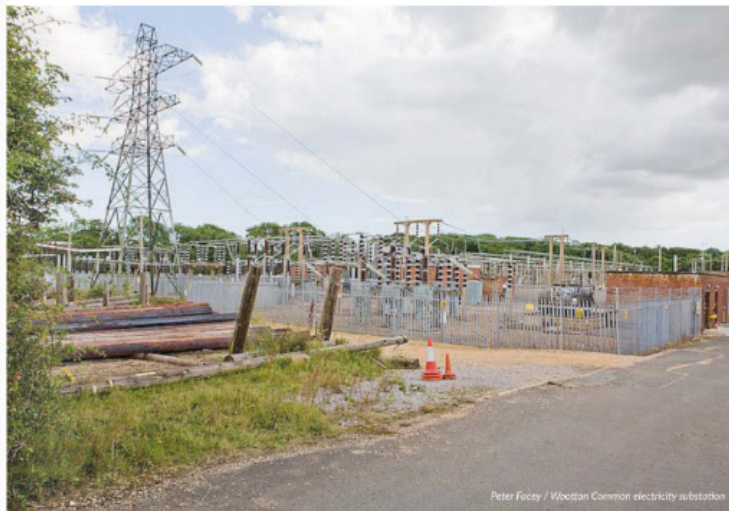
Peter Feely / Woodson Common electricity substation
